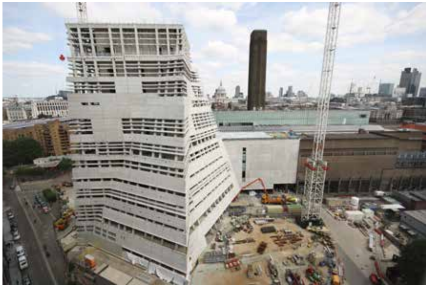
Tate Modern's extension took shape over 2013/14 and the external structure is now almost complete.
